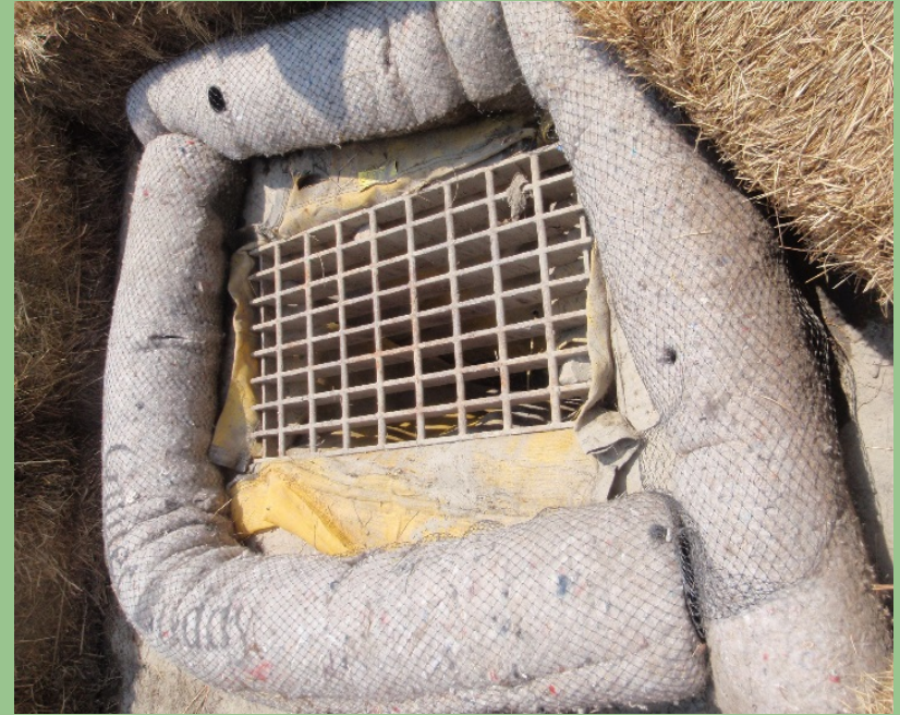
implementation of control measures
