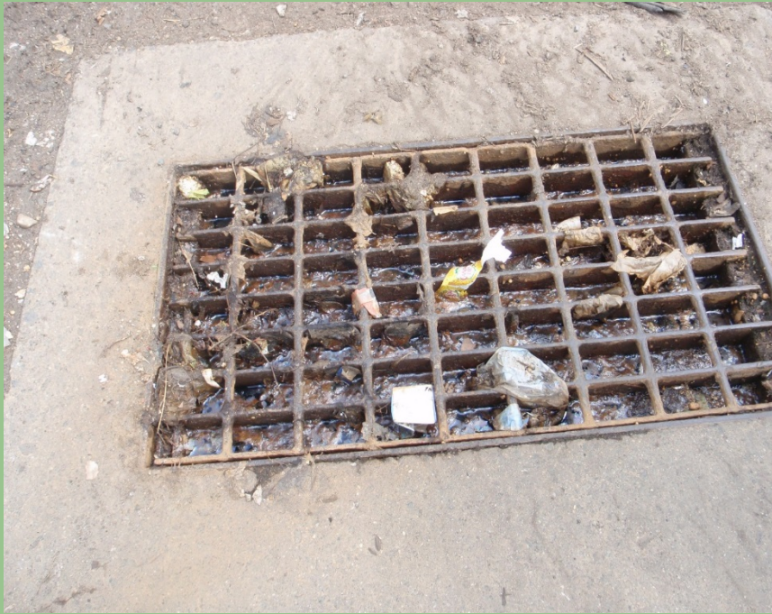
clogged catch basin
